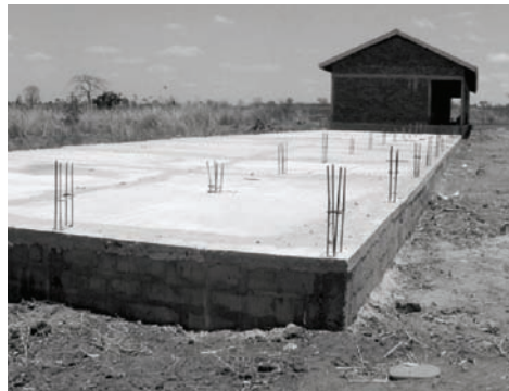
September 2009: The shell of the first classroom is complete and the foundation is poured for another.
